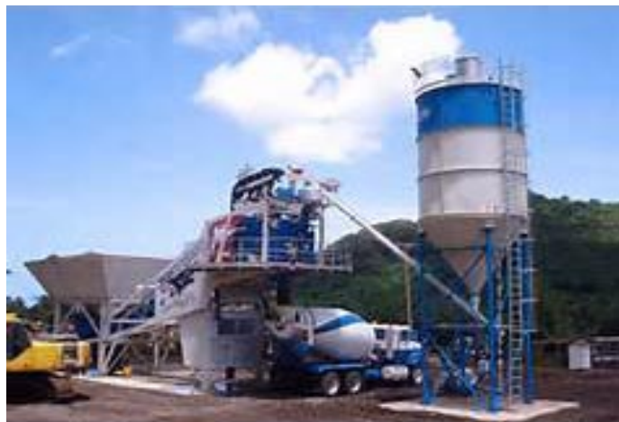
Figure 400-16 — CONCRETE BATCH PLANT
