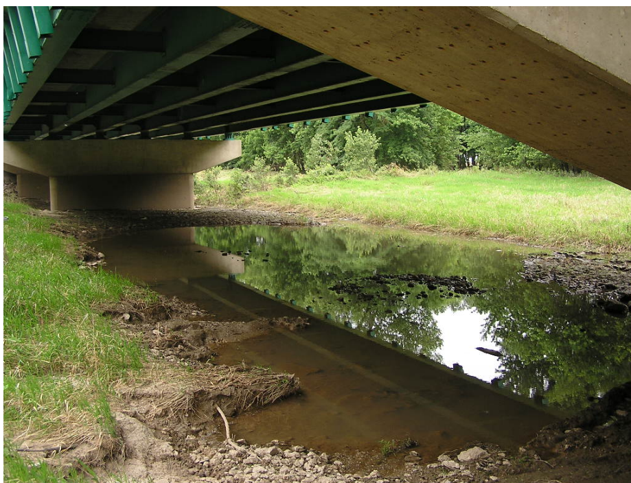
Figure 10-202 Overbank contraction scour hole submerged
