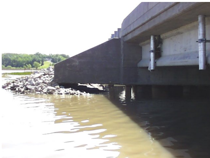
Scour of bridge abutment and approach embankment Figure 10-304.01c
