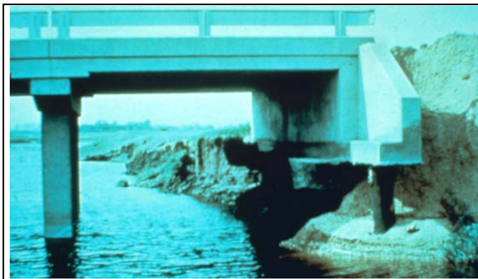
Scour of bridge abutment and approach embankment. Figure 10-304.01b
