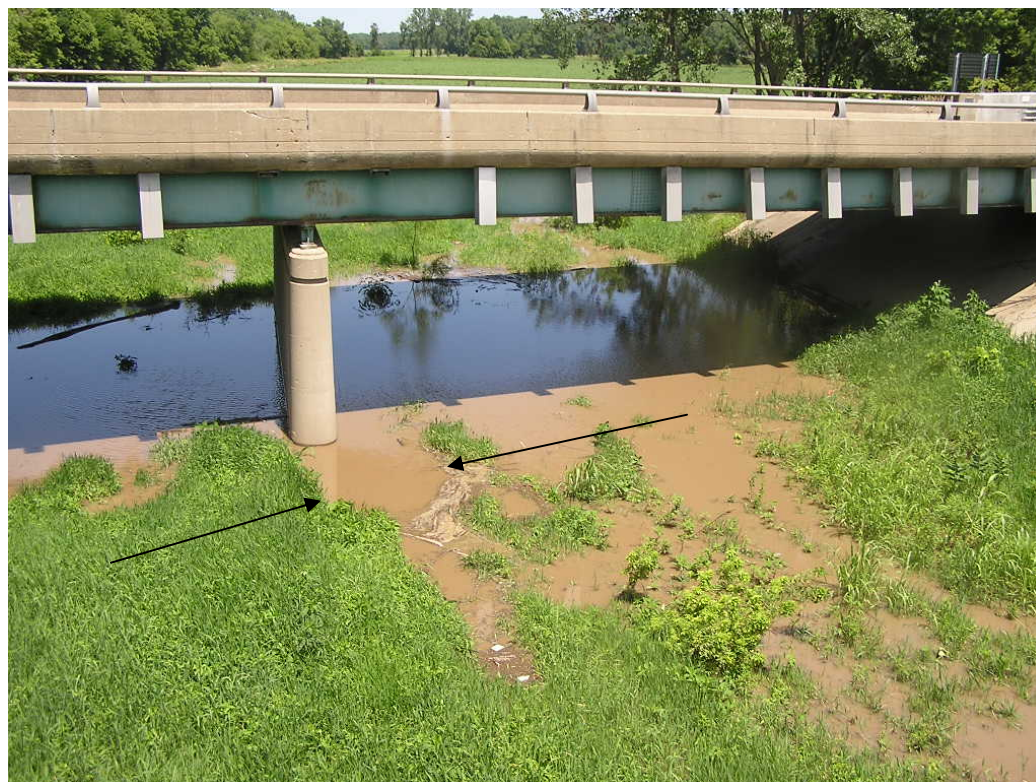
Pier Scour Figure 10-303
