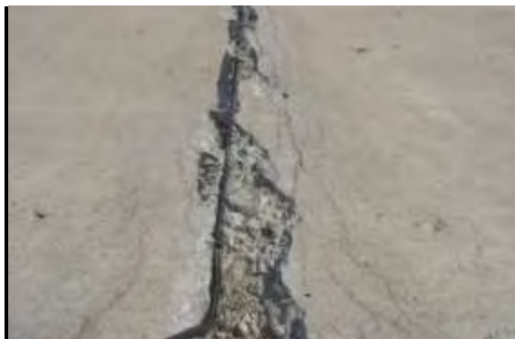
Severe D-Cracking - A well defined cracking pattern with a significant amount of loose or missing material.
