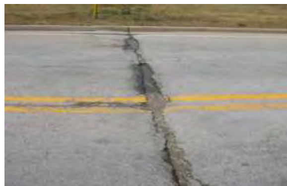
Severe L&T Cracking - Cracks are wide, have significant spalling, or are accompanied by adjacent moderate severity random cracking.
