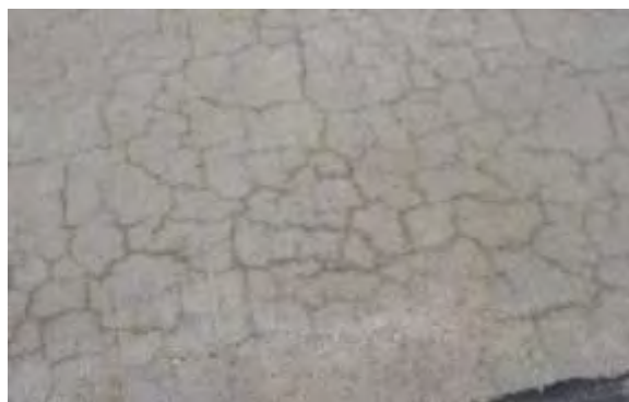
Light Surface Distress - Very clear cracking pattern on the surface, where cracks appear tight and shallow; no scaling.
