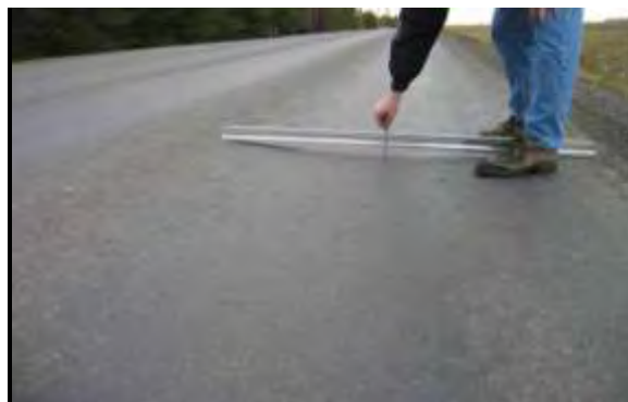
Moderate Rutting - Rut depth approximately between ½ inch and 1 inch (12.7 mm and 25.4 mm) in a given location.
