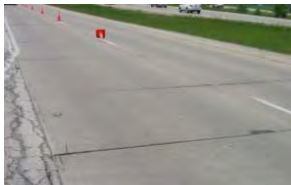
Light Faulting - Faulting is visible and measures approximately less than ¼ inch (6.4 mm) at a given location.
