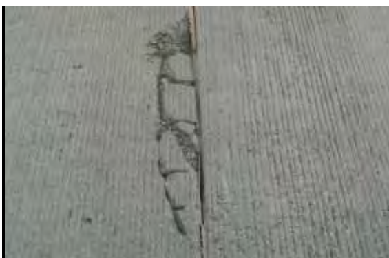
Severe Spalling - Considerable wear and loss of material at the joint or crack; ride quality is affected.
