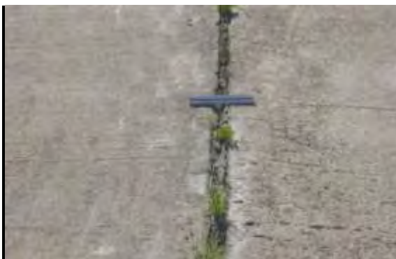
Severe Joint Seal Damage - Sealant is mostly missing, oxidized (no longer pliable), split, or is lost all adherence; sealant is no longer performing its intended function.
