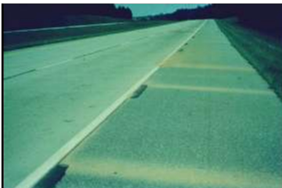
Severe Pumping - Excessive amounts of staining. Additional indications may include faulting or the erosion of shoulder pavement from applied pumping forces.
