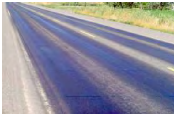
Severe Bleeding – Bleeding covers much of the pavement surface and is relatively thick.
