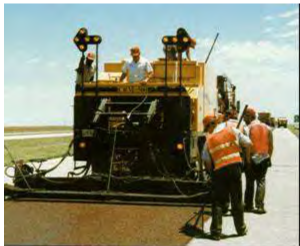
Step 6. Slurry placement. This photo shows the placement of material using a microsurfacing spreader box. This material should be placed within 12 days of the placement of the chip seal.
