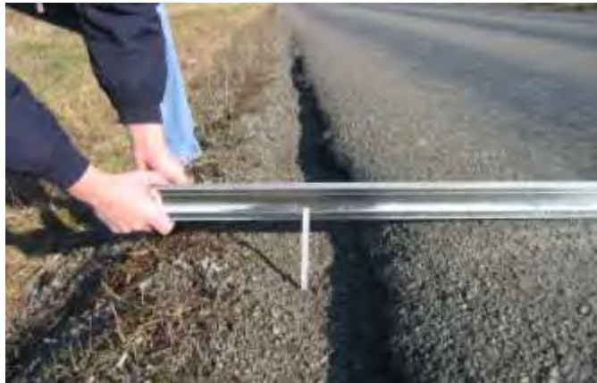
LANE-SHOULDER DROP OFF
