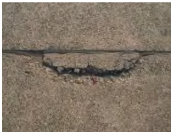
Light Spalling - Slight wear along the joint or crack, with minimal loose or missing pieces.
