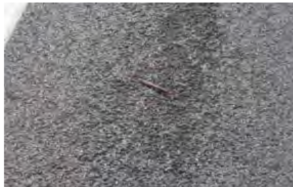
Moderate Weathering/Raveling - Some aggregate loss resulting in an overall rough pavement surface with some localized pitting.
