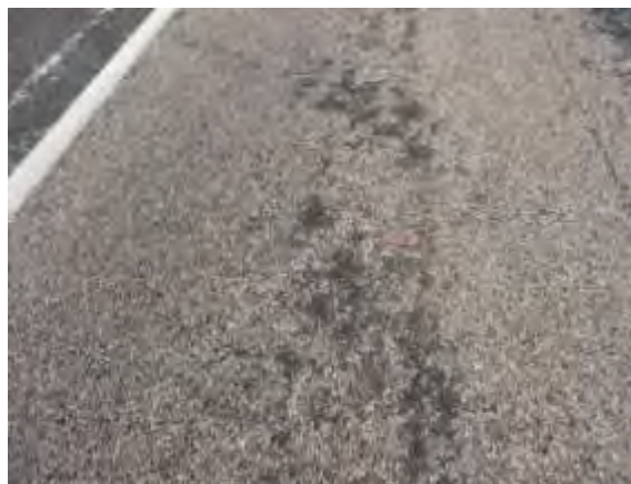
Light Bleeding – Small or isolated areas where asphalt material has pooled on the pavement surface.
