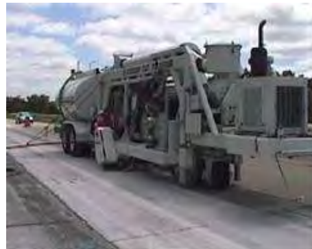
Steps 8 & 9. Diamond grinding & joint sealing. Final steps often consist of diamond grinding and joint sealing.
