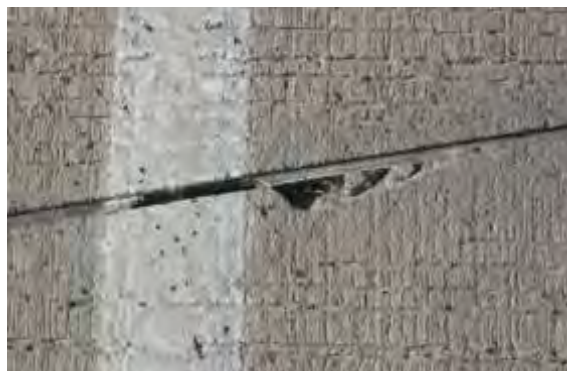
Light Joint Seal Damage - Only localized areas of the sealant are damaged.
