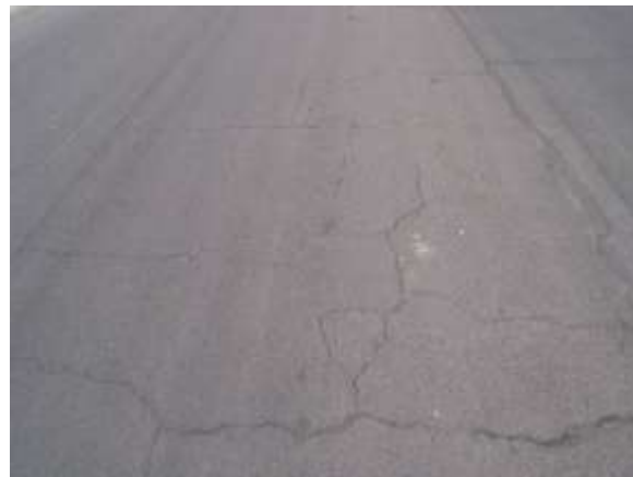
Light Block Cracking – Tight cracks or sealed cracks with the filler in good condition.
