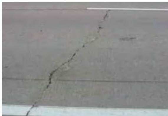
Moderate Transverse Cracking - Wider cracks with some spalling or faulting.
