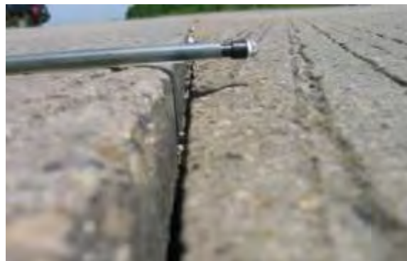
Severe Faulting - Faulting is greater than approximately ½ inch (12.7 mm) at a given location.
