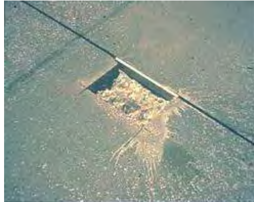
Step 4. Joint preparation. It is important to maintain the existing joint reservoir during construction.
