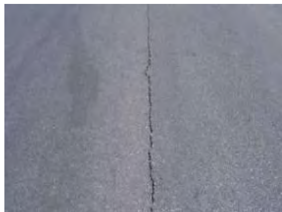
Light L&T Cracking - Tight cracks or sealed cracks with the filler in good condition.
