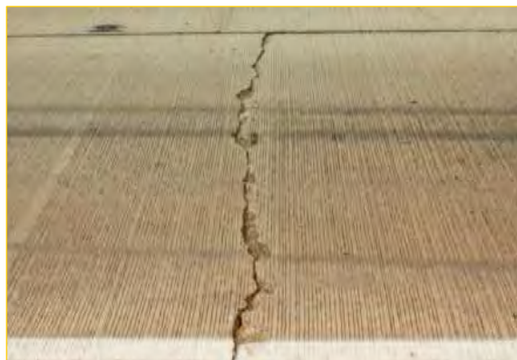
Severe Transverse Cracking - Cracks that exhibit movement accompanied by discernable spalling or faulting.
