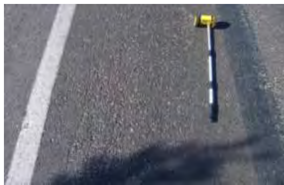
Light Weathering/Raveling - Some aggregate loss from the pavement surface with little or no pitting.
