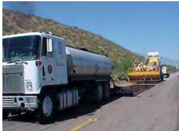
Steps 2 & 3. Binder and aggregate application. The asphalt binder is applied to the surface with a distributor truck. A self-propelled, pneumatic-tired, motorized unit has a hopper on the front where the chips are dumped.
