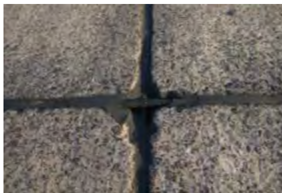
Moderate Joint Seal Damage - Portions of the sealant are missing, oxidized (no longer pliable), split, or have lost adherence.
