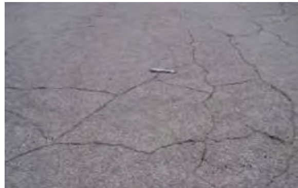
Moderate Block Cracking – Cracks have opened up, exhibit a small amount of spalling, or have adjacent random light cracking.
