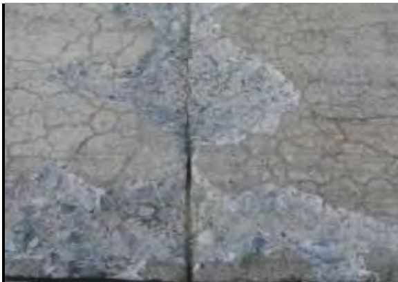
Severe Surface Distress - Extensive material loss (scaling).
