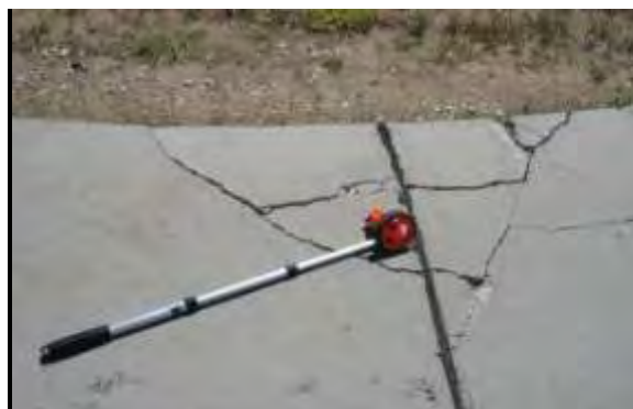
Severe Corner Breaks - Crack is heavily spalled; corner is broken into two or more pieces, is faulted, or moves under load.
