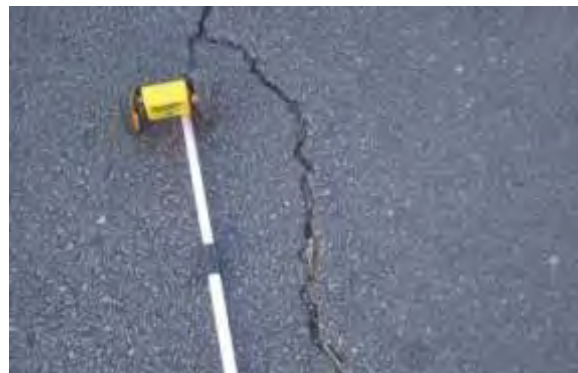
Moderate L&T Cracking - Cracks have opened up, exhibit a small amount of spalling, or have adjacent random light cracking.
