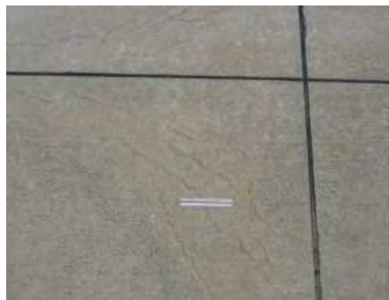
Light D-Cracking - Tight cracks with no loose or missing pieces and no patching in the affected area.
