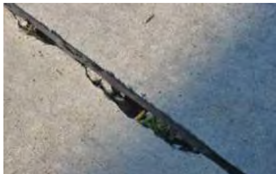
Moderate Spalling - Shallow but discernable wear at the joint or crack, with loose pieces that can be removed easily or are missing.
