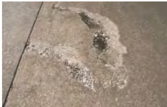
Moderate Surface Distress - Cracks have opened up and/or there is some material loss (scaling) on the pavement surface.
