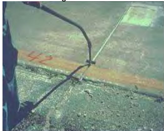
Steps 7 & 8. Curing & joint sealing. The final steps include texturing and providing adequate curing.
