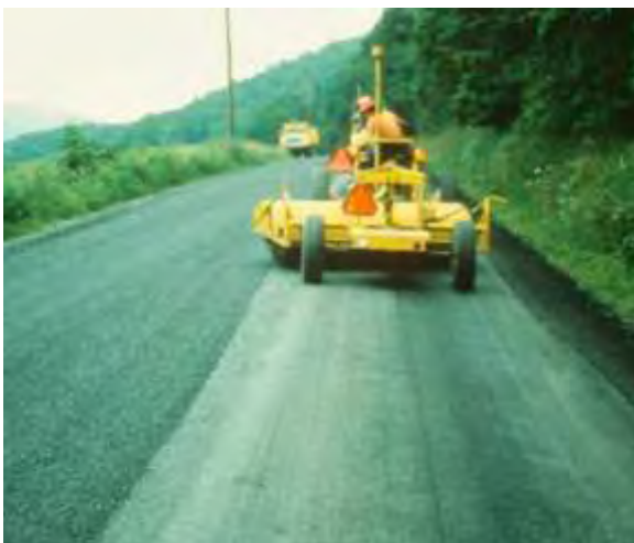
Steps 4 & 5. Rolling and brooming. After the application of the aggregate, the surface is rolled with pneumatic-tired rollers and broomed to remove excess aggregate.
