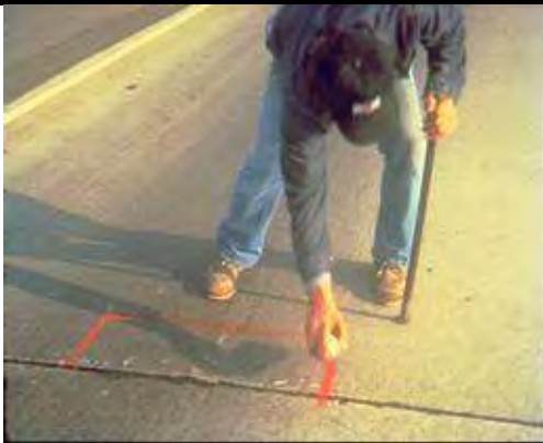
Step 1. Repair boundary marking. Determine extent of unsound material, and mark repair boundaries.
