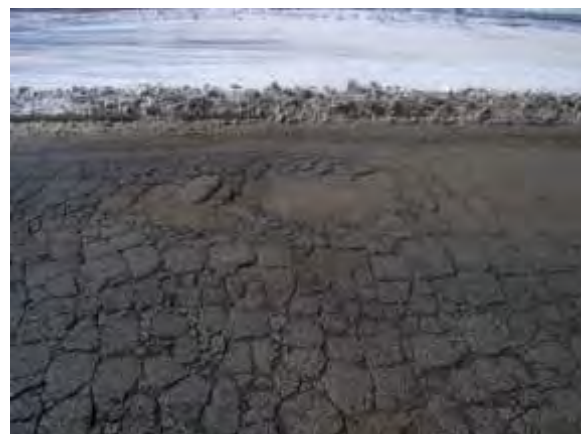
Severe Alligator Cracking - Cracks are wider and pieces are spalled and show movement under traffic loads.
