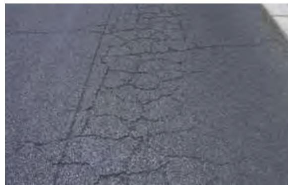
Moderate Alligator Cracking - Cracks are interconnected and may be slightly spalled, but are stable.
