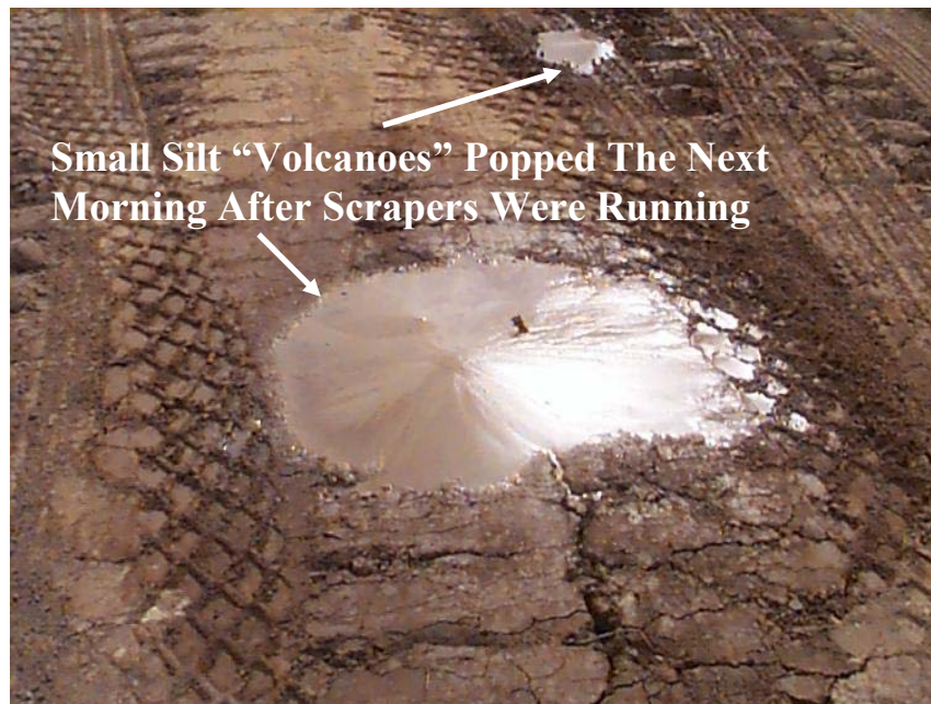
Figure 2. Repeated truck/equipment loads will draw moisture up to the surface of silty subgrade soils (pumping).
