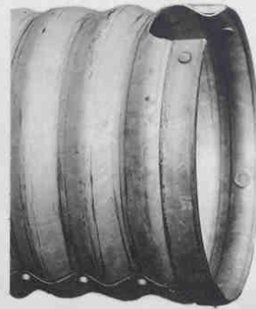
Figure 13 - Galvanized Bar Satisfactory
