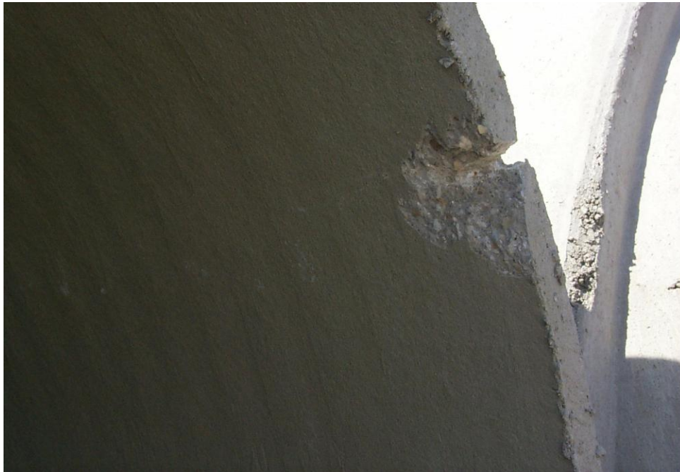
Figure 16 - Chipped Spigot – May be repaired
