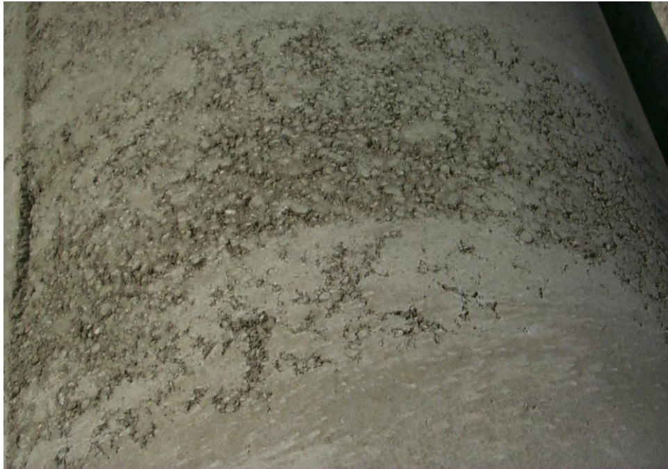
Figure 15 - Honeycomb Inside – Sufficient to reject
