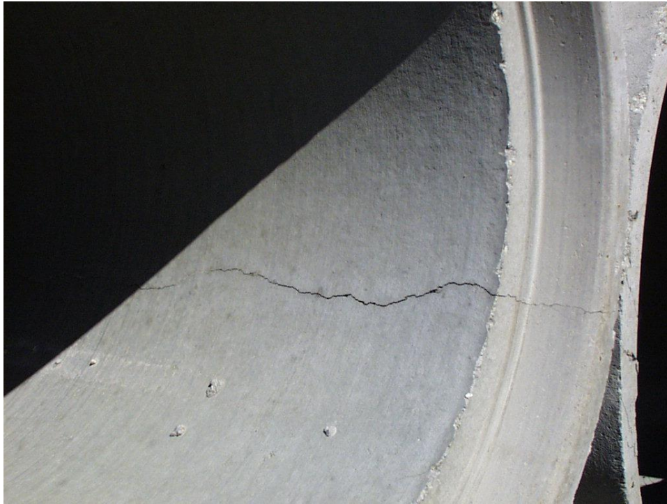
Figure 1 - Crack Through Wall – Cause for rejection
