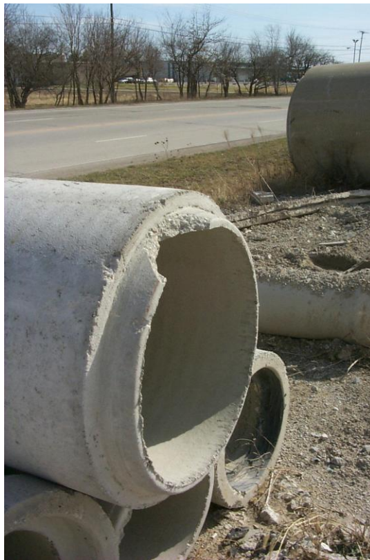
Figure 8 - Chipped Spigot – May be repaired.
