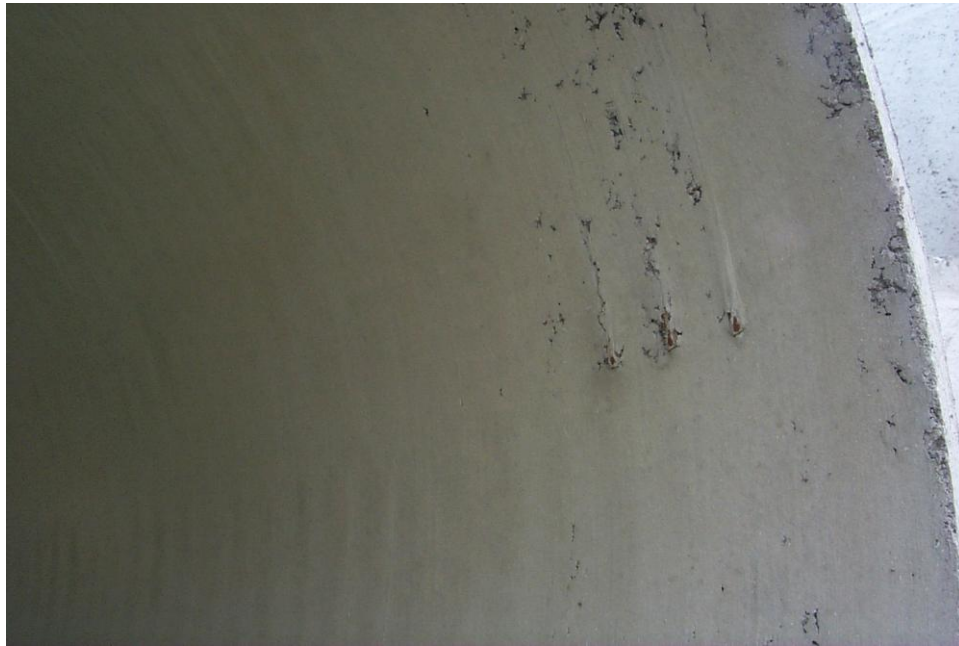
Figure 18 - Exposed Wire Inside – Cause for rejection
