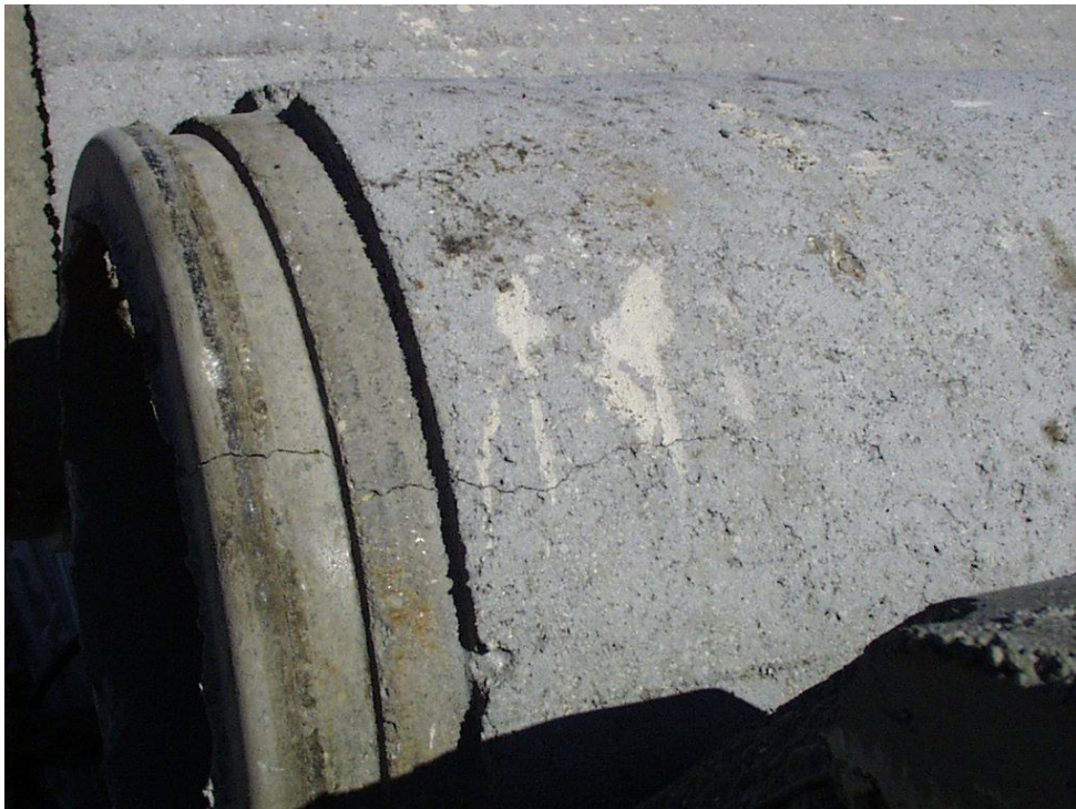
Figure 2 - Crack Through Wall – Cause for rejection
