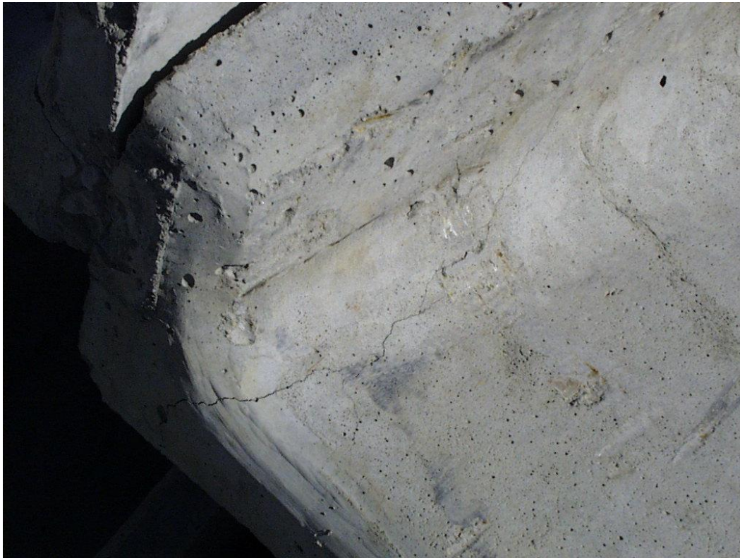
Figure 6 - Cracked End Section – Cause for rejection
