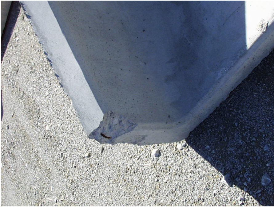
Figure 5 - Chipped End Section – May be patched
