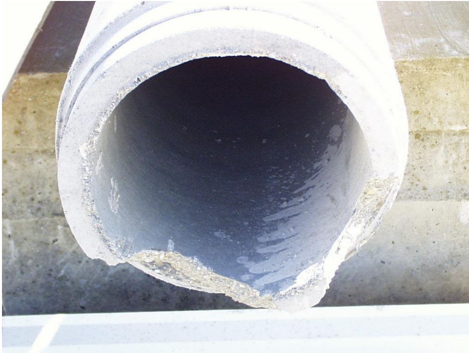
Figure 7 - Broken Spigot – May not be repaired
