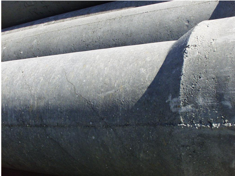
Figure 3 - Cracks – Cause for rejection.
