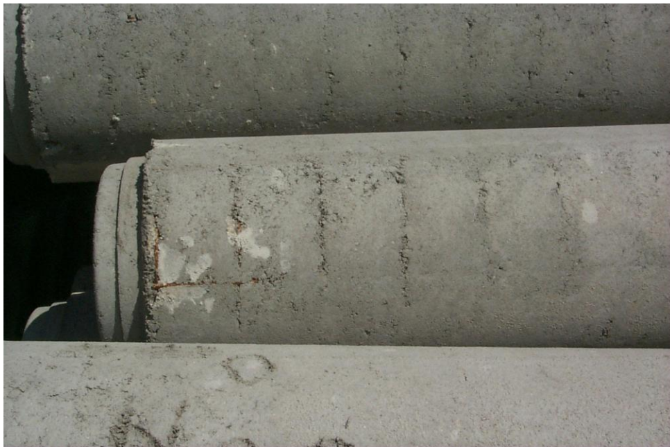
Figure 20 - Exposed Wire – Cause for rejection
