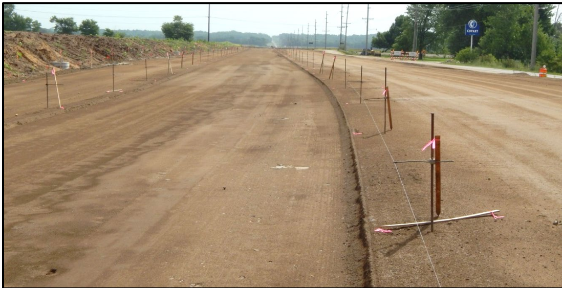
Figure 15. Photo of Fly ash modified Improved Subgrade is fine graded and ready for paving.
