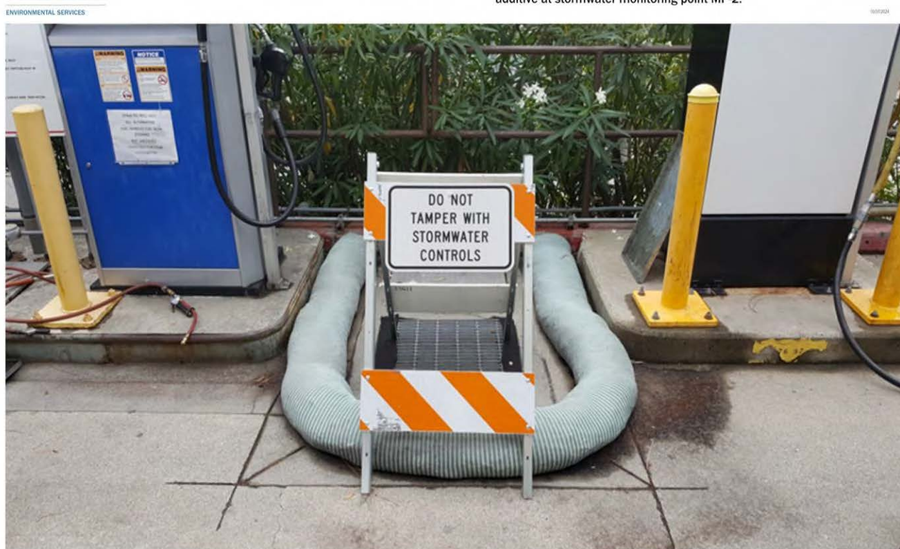
Figure 4-2. Compost filter sock and drain inlet filter fabric at stormwater monitoring point MP-2.
